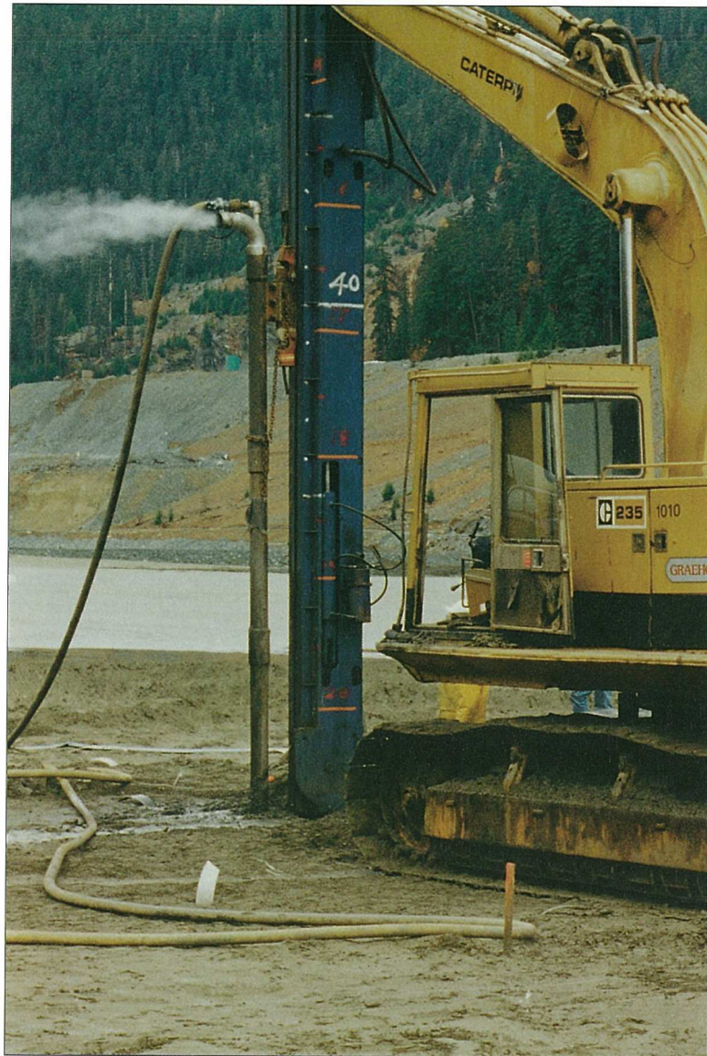
Photograph 7. Vibro-Drain operating at Myra Falls showing water discharge from filter/drain module exhaust
