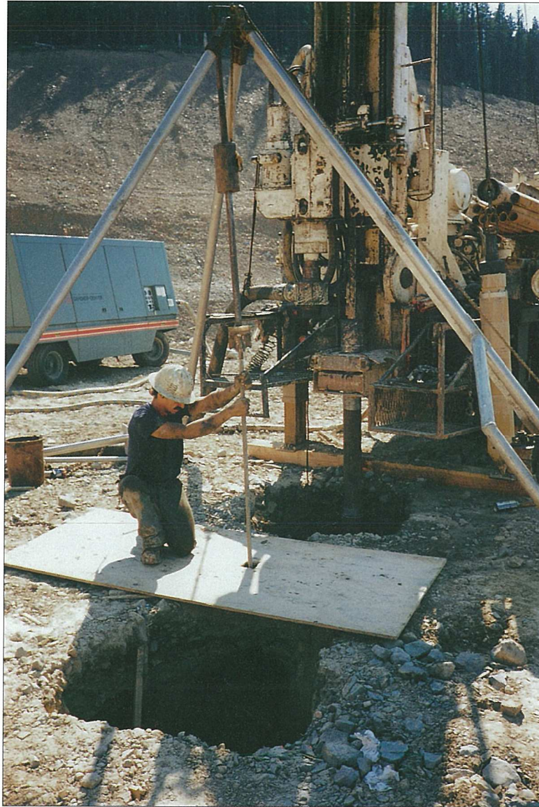
Photograph 5. Craters in Blackdome tailings dam u/s slope at locations of two Vibro-Drain treatment axes
