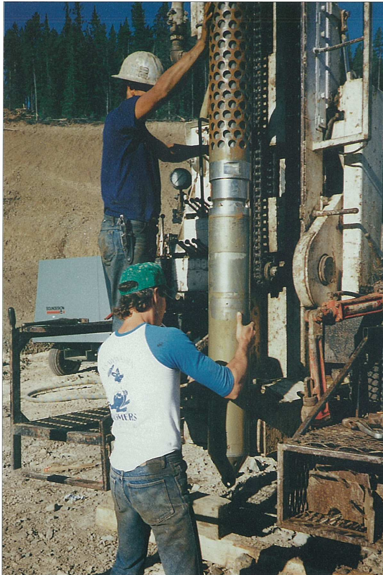
Photograph 1. Vibro-Drain equipment at Blackdome Mine showing filter/drain module (above) and vibrator (below)
