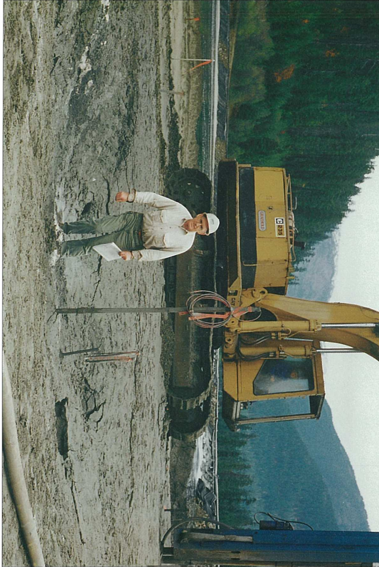
Photograph 8. Surface settlement and cracking of Myra Falls test pad at location of 7-point treatment array
